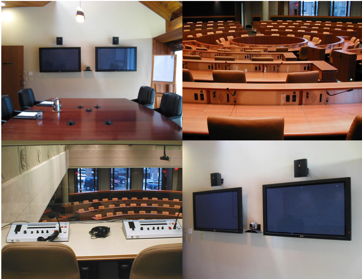
High-tech installations at IACC-member facilities. Upper left and lower right: Boardroom and flat panel displays with HD wide-angle camera and point-source speakers for video-teleconferencing at a private facility in Racine, Wisconsin. Upper right and lower left: View across auditorium with delegate communications panel in foreground and view from simultaneous interpretation booth at SFU Morris J Wosk Centre for Dialogue in Vancouver, British Columbia.
